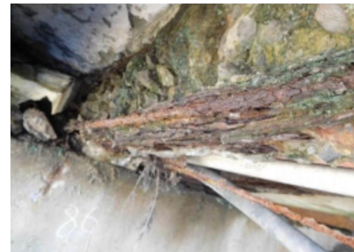
纵梁底面露筋锈蚀
