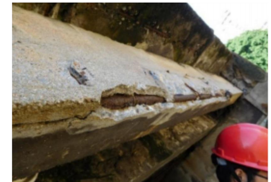
纵梁底面露筋锈蚀
